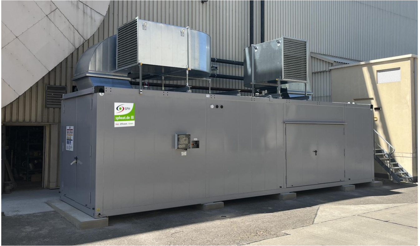
Figure 1: Outdoor installation of two-stage HP system embedded in a container solution
