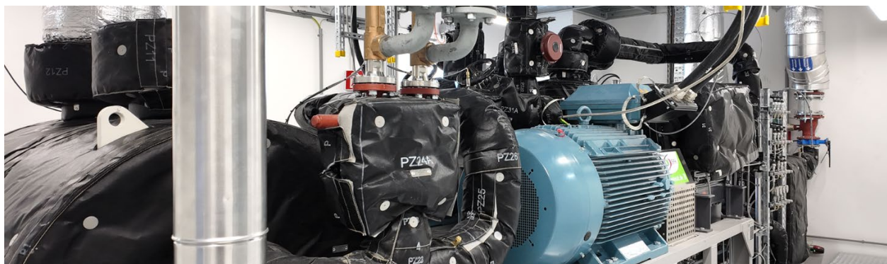
Figure 1: NEFI AHEAD Heat Pump at Takeda pharmaceutical production site in Vienna, Austria (photo: Takeda)
